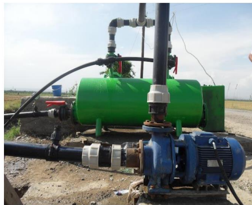
Fig. 2 Pumps in the system
