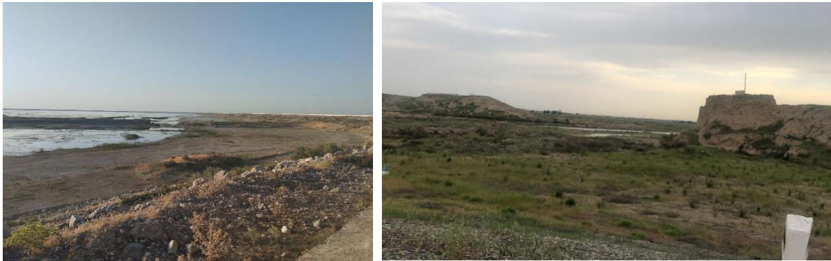
Figure 1. The collapse that occurred in the dam section between pickets PK57+00-PK60+00 of the Sardoba reservoir
